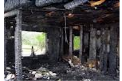
Results of a kerosene heater fire
